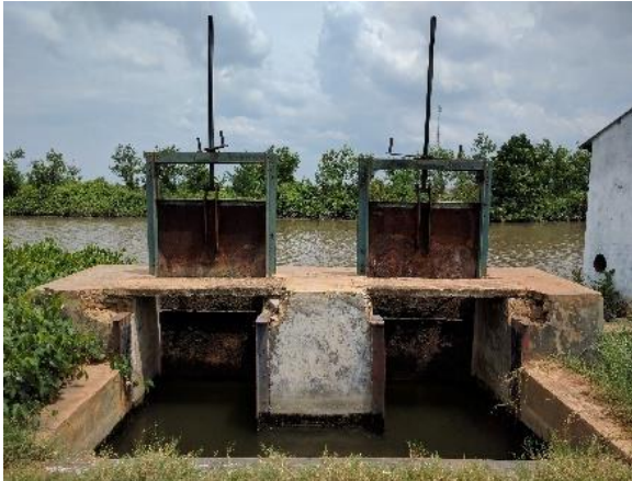
Figure 4, intakes are open during the day when drainage using gravity is possible to river Meduri
