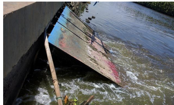
Figure 7 and 8 are pictures made by the two upper red dots. During high tide of the Java sea, water is able to flow into the fishponds. Wooden shields are installed, shown in figure X, to prevent to water from flowing in. As a result of bad maintenance these shields cannot block water anymore.
